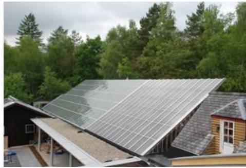
20 kW Solar Roof at the Centre for Alternative Technology, Machynlleth, Wales
